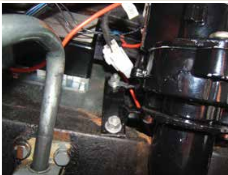
Photo EZ power-3 Installation showing the additional bracket made to anchor the power unit at the new steering-column flange. The power computer is shown mounted on the fire-wall (behind the battery).
