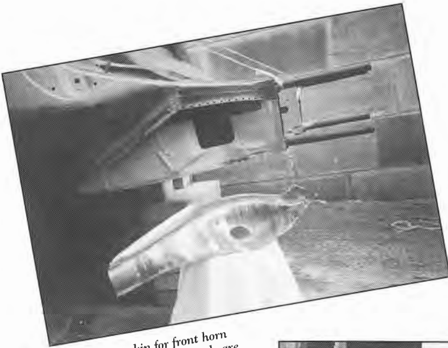
New inner skin on front horn ready for welding, front horns should be braced to prevent movement during welding.
