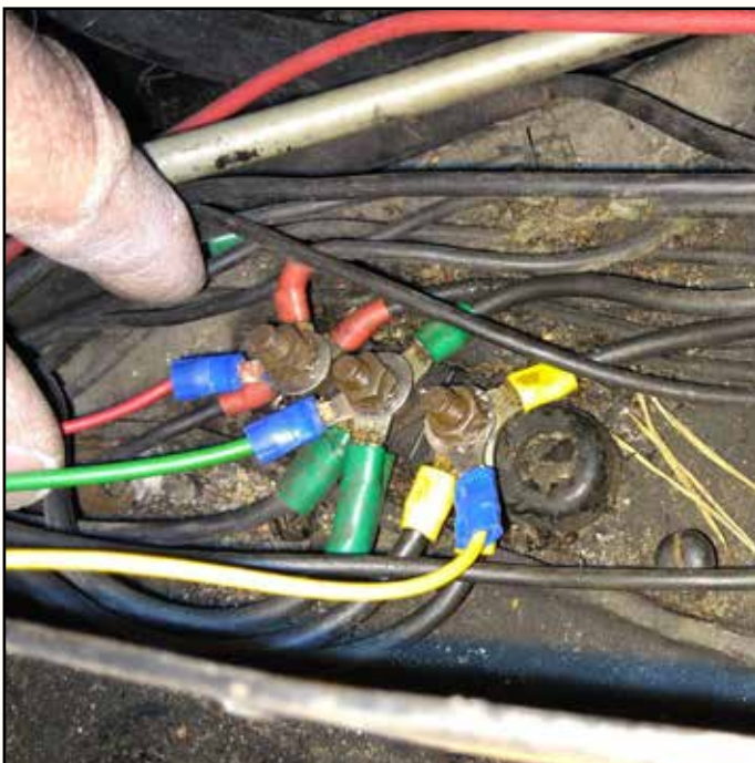
The terminal block on the left "jambonneau". Yellow cable lugs and yellow cable: Dipped beam. Green cable lugs and green cable: High beam Red cable lugs and red cable: Sidelight
